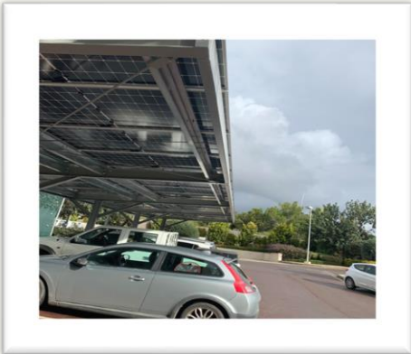
PV PANELS COVERED PARKING
